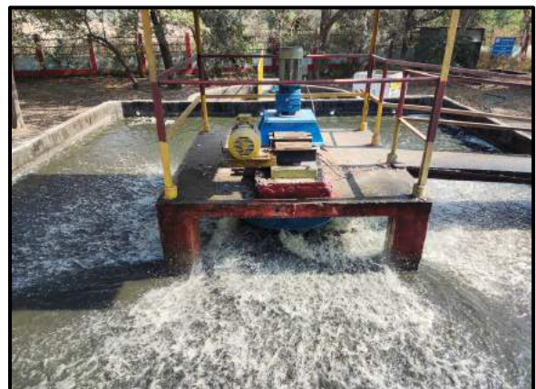
Surface Aerator at Treatment plant, Bhalar Township, Wani North Area
