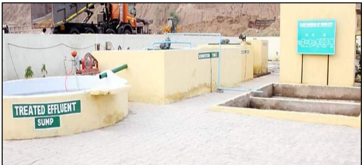
Effluent Treatment plant, Amalgamated Inder-Kamptee OC, Nagpur Area
